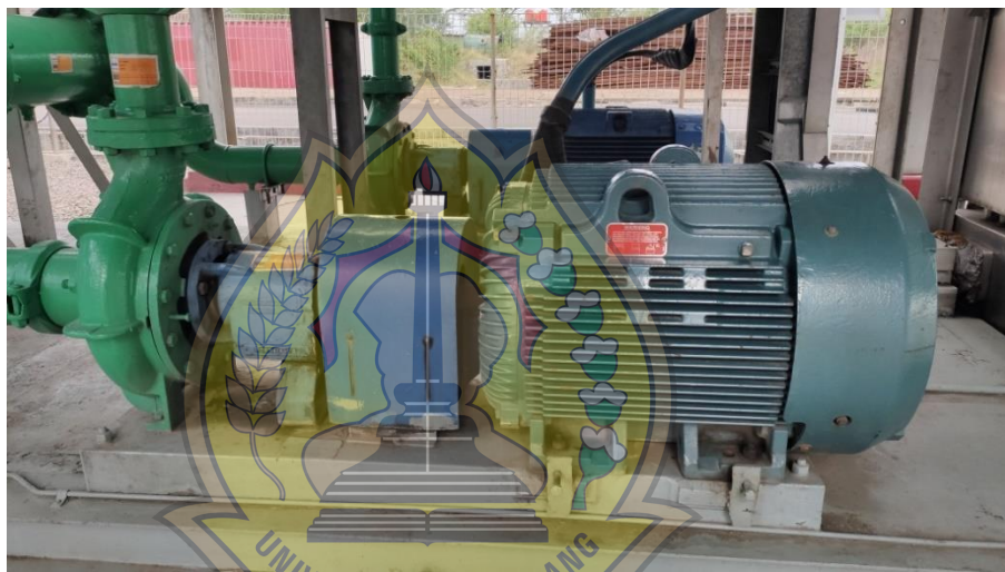
Gambar 2. 3 Motor Water Pump Cooling Pump (Dokumentasi Pribadi)
